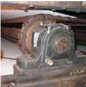
Pulp & Paper Industry, Canada. LabTecta-PB™ installed on a dryer roll (Case Ref: 3369)
