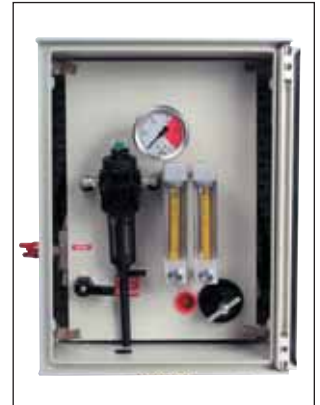
Above: All instruments are inside the cabinet
