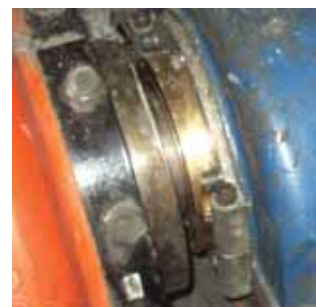
LabTecta-RDS-AX™ installed on a primary air fan (Case Ref: 3389)
